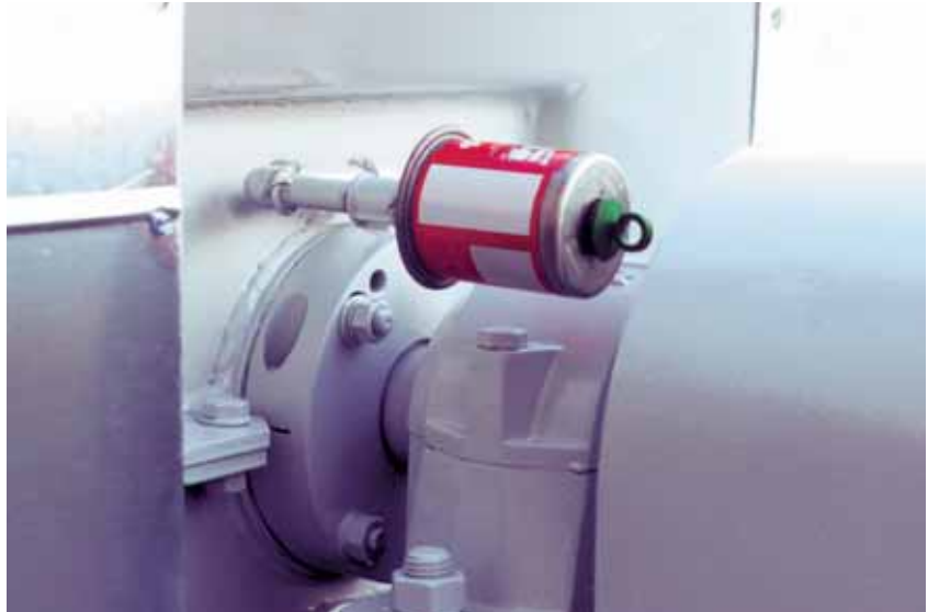
Shaft seal with grease dispensers
